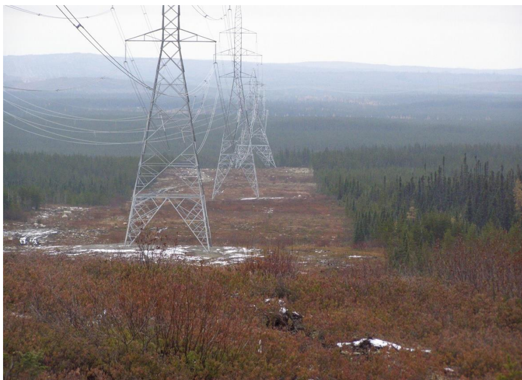
Figure 6 - Power line at Rose Site
