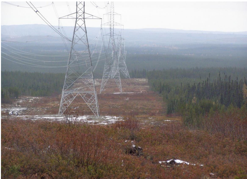
Figure 6 - Power line at Rose Site
