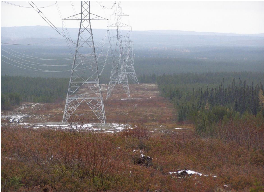
Figure 6 - Power line at Rose Site
