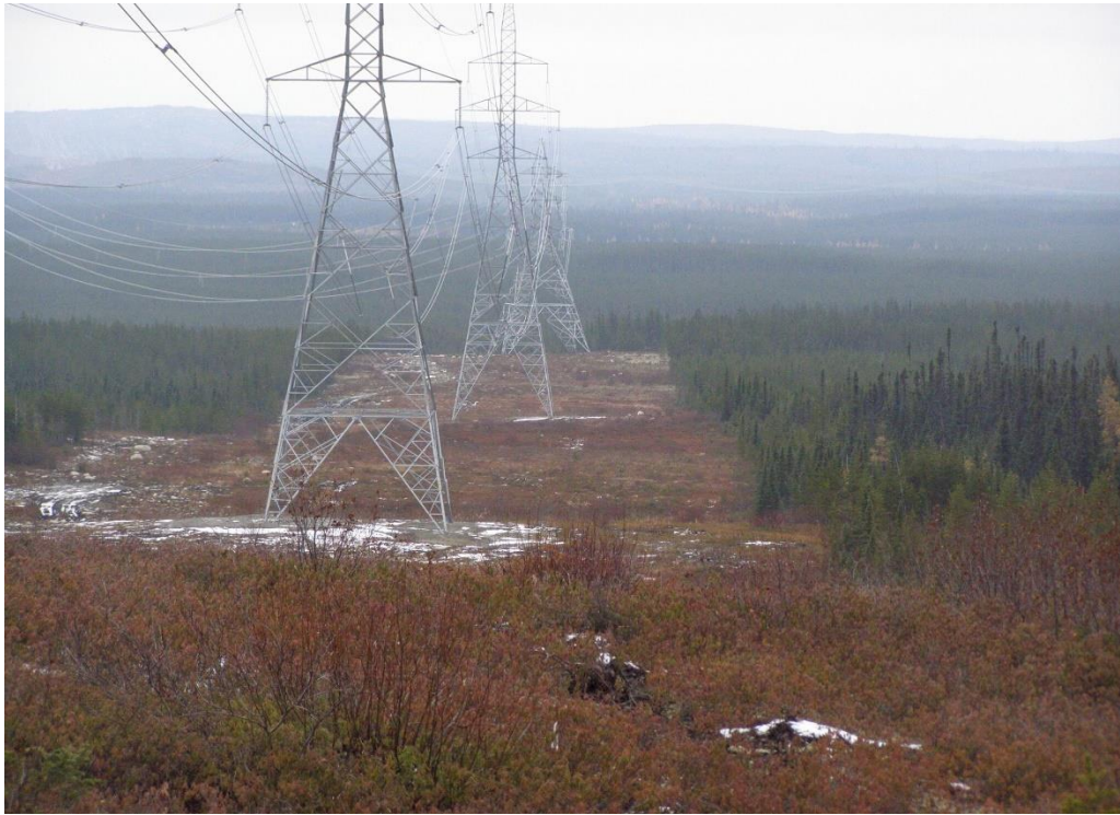
Figure 6 Power Line at Rose Site
