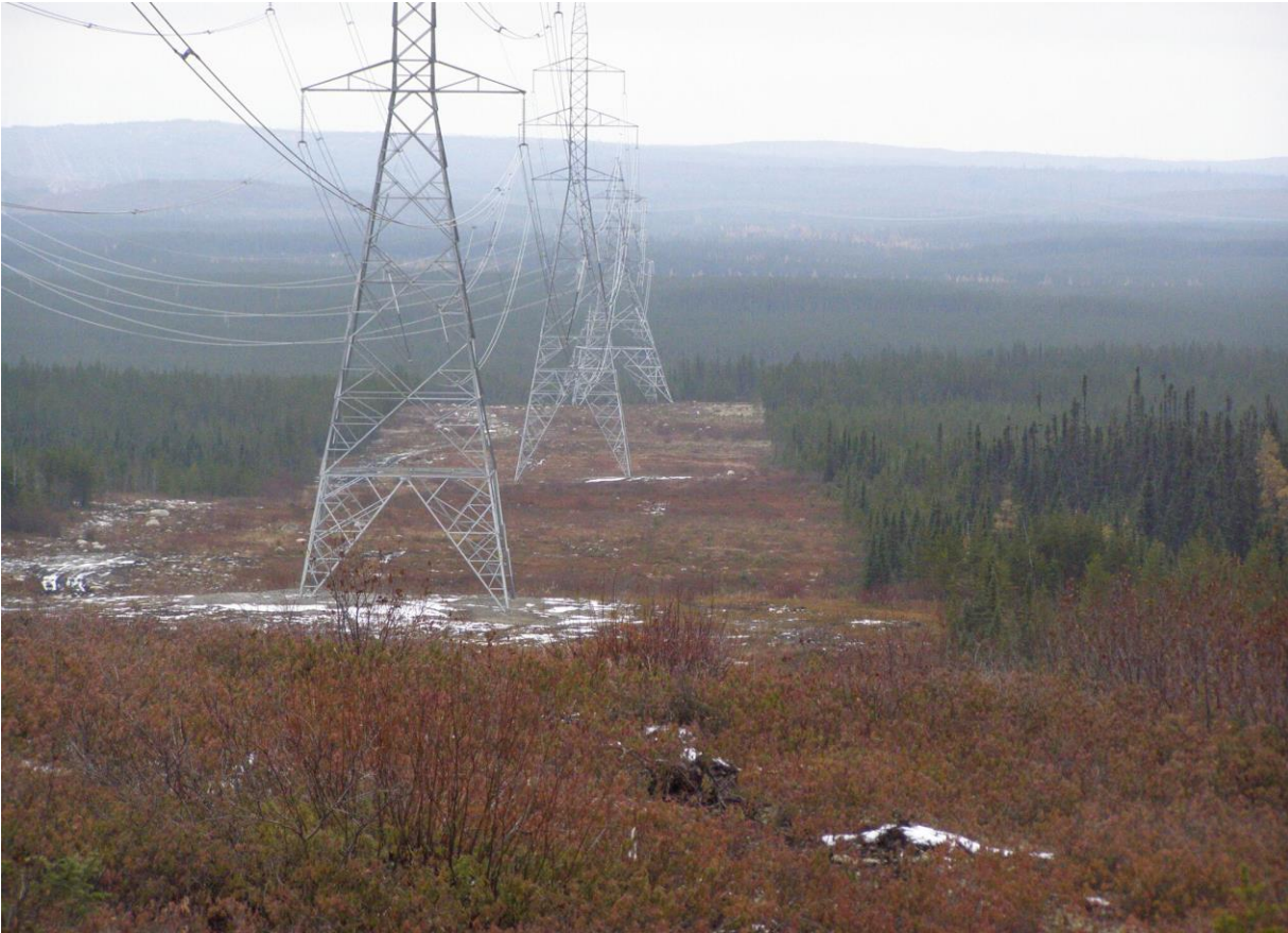
Figure 6 Power Line at Rose Site
