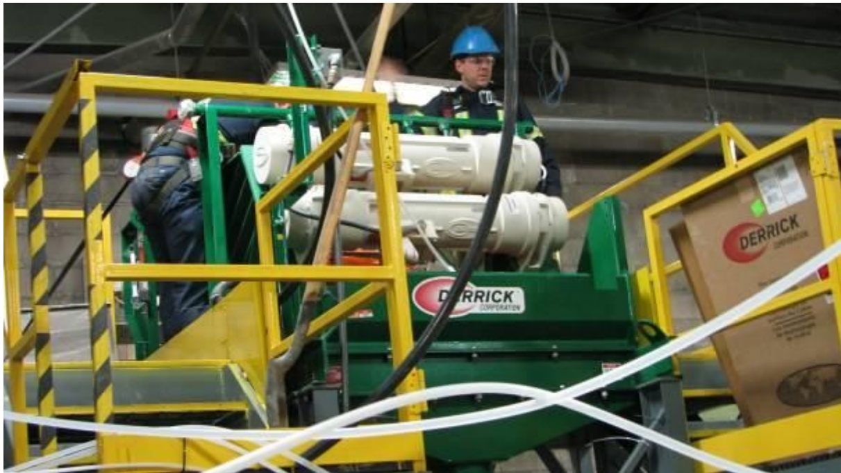
Figure 2 - Ball Mill & Derrick Screen. Overs from Derrick feed Ball Mill
